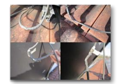
Damaged DC cables due to aging
