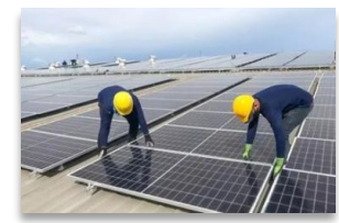
During installation and O&M, personnel are prone to contact with high voltage.
