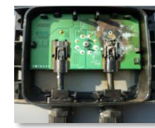
Unreliably-welded PV junction boxes
