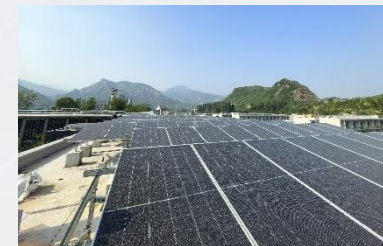
Factory Rooftop Plant @Beijing 26% more modules installed in shaded areas.
