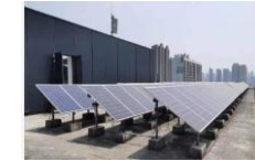
Parapet wall/Staircase enclosure/Billboard
