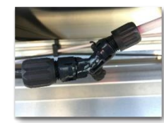
Incompatible connectors or unreliable connections
